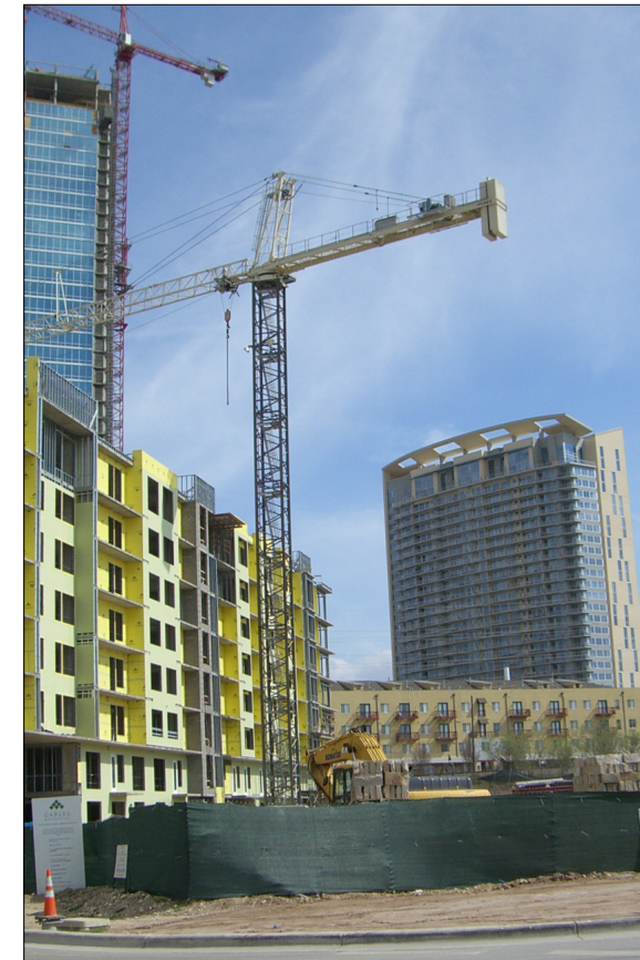
Gables on 5th Street in the foreground is under construction. In the background: The Spring (under construction and Monarch (completed in 2007)
